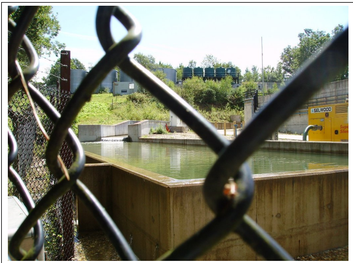
Figure 4. The North Ponds Water Management System at AWE Aldermaston on 21st July 2007 – the day after the floods. Holding tanks in the system are full and water can be seen overtopping the concrete wall of the lower tank and draining away underneath the perimeter fence of the base.
