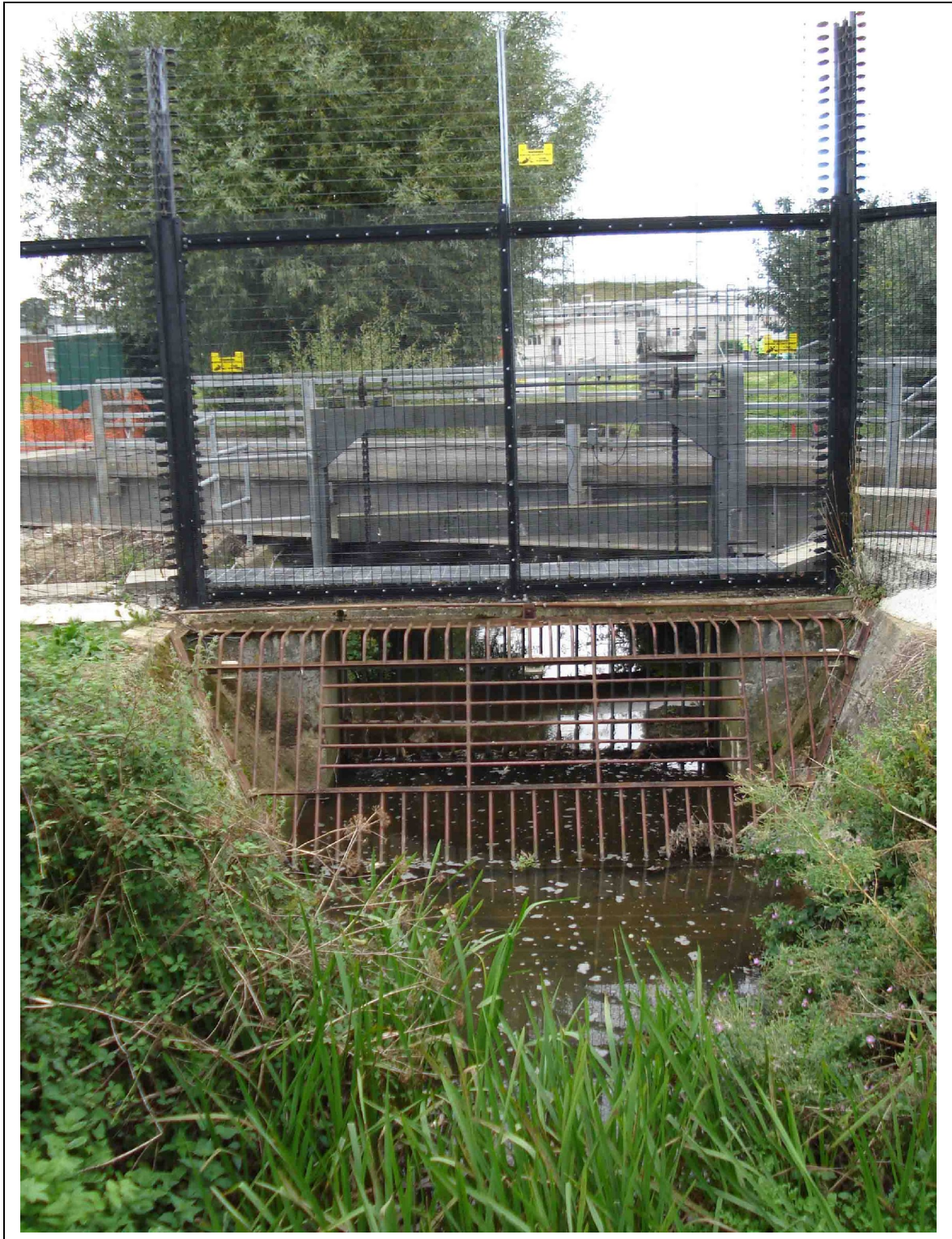
Figure 2. The Burghfield Brook emerges from under the security fence on the Eastern perimeter of the AWE Burghfield site. On 20th July 2007 flood water from the brook, which flows around the edge of the site, overwhelmed buildings in the nuclear licensed site at AWE Burghfield.
