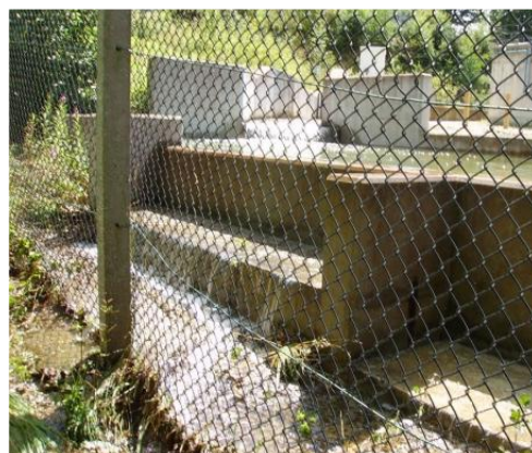
Flood water overflowing from North Ponds radioactive wastewater store at AWE Aldermaston
