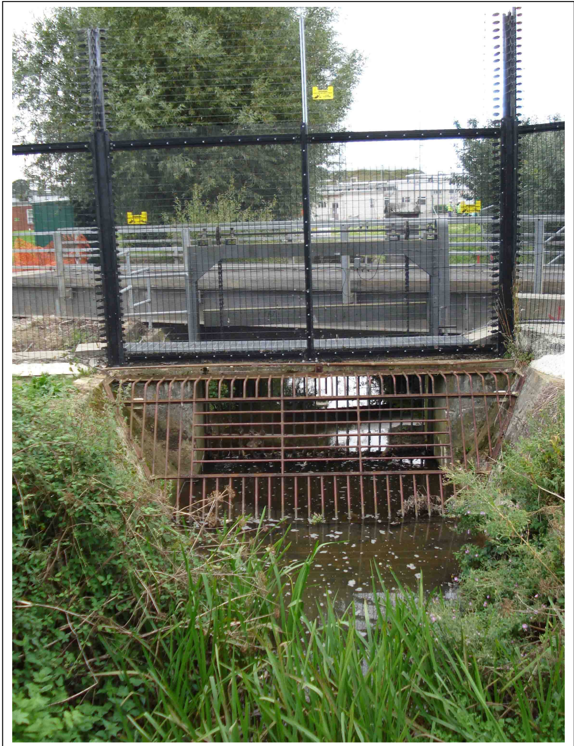
Figure 2. The Burghfield Brook emerges from under the security fence on the Eastern perimeter of the AWE Burghfield site. On 20th July 2007 flood water from the brook, which flows around the edge of the site, overwhelmed buildings in the nuclear licensed site at AWE Burghfield.
