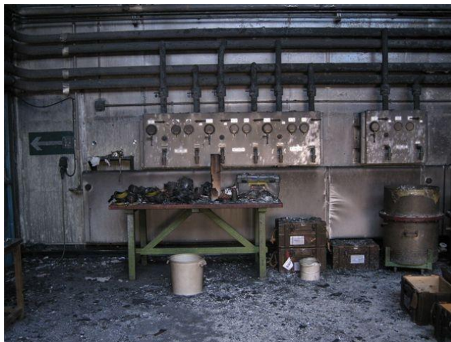
Internal view of the building after the fire
