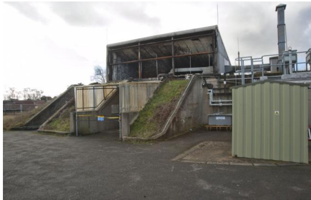
External view of the building after the fire
