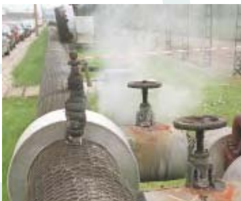
A section of the 60 kilometres of steampipe at AWE Aldermaston.
