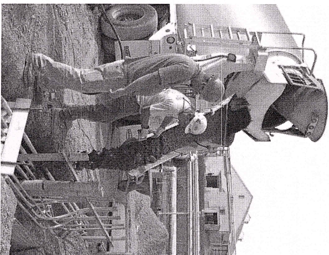
Workers perform the first concrete pour of duct banks for the Purification Facility.
